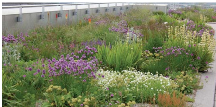
Moorgate Crofts Business Centre, Rotherham with a 'semi-intensive' green roof designed by Nigel Dunnett. It has a substrate depth of 8cm, supplied by Alumasc, and a wide range of species is used, many of which are normally associated with domestic rock gardens
